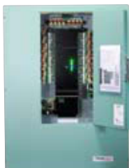
Lighting Control Panel
