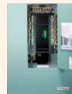
Lighting Control Panels
