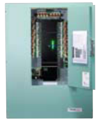
Lighting Control Panel
